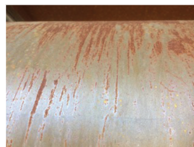
Surface rust on roller
